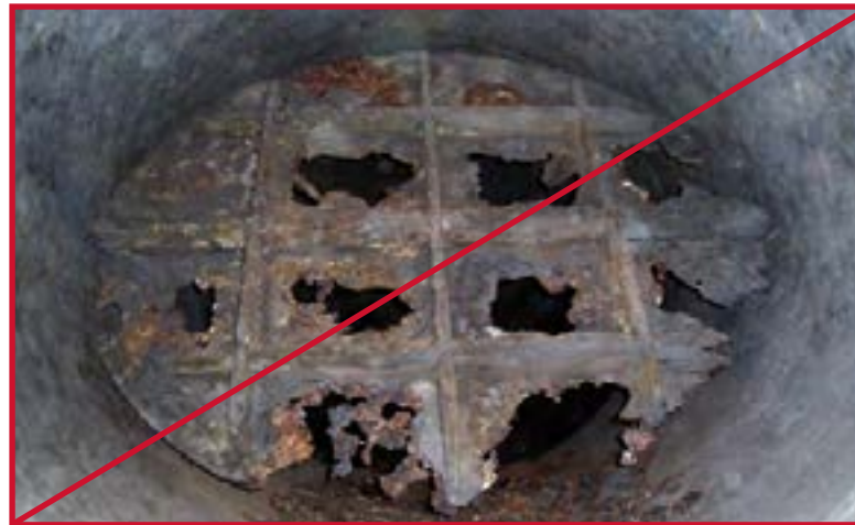
Fire damper that will not pass inspection
