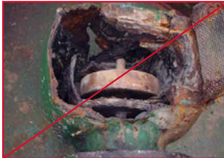
Vent head that will not pass inspection.
