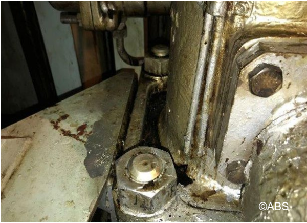
Oil leakage from main engine fuel pump
