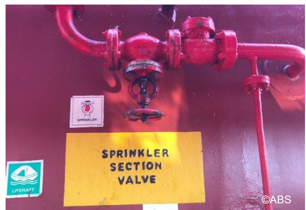
Paint room sprinkler system not in operation due to isolation valve stuck
