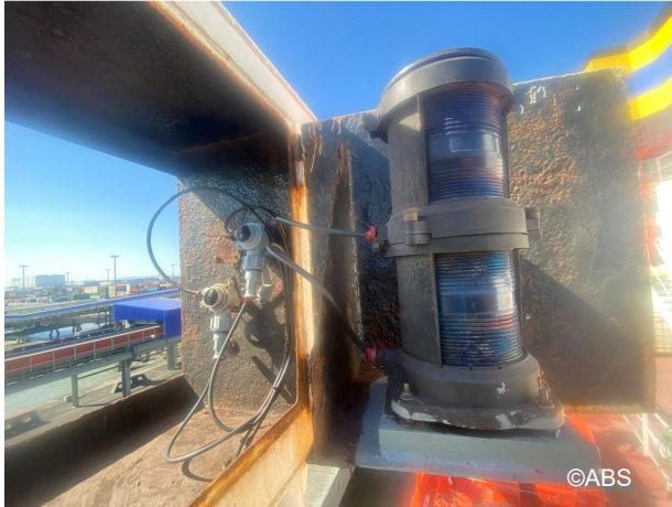
Navigation light not properly mounted and mounting screw missing
