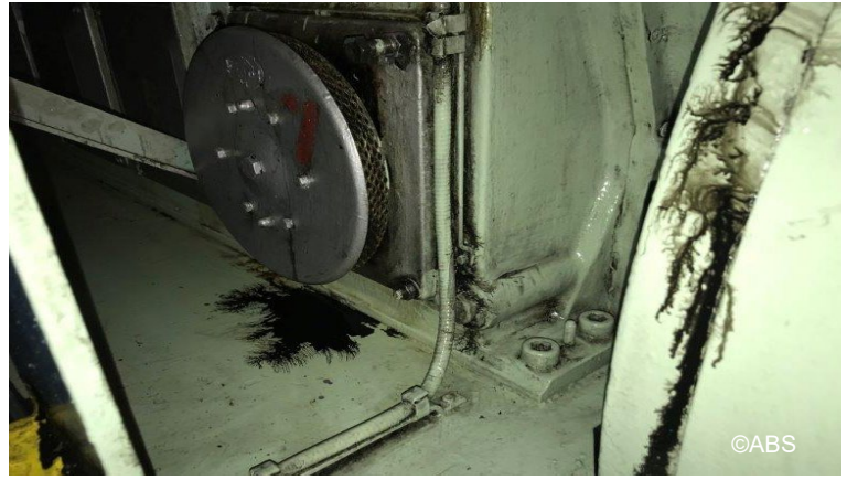
Oil leakage from generator engine crank case explosion door and fly wheel end seal
