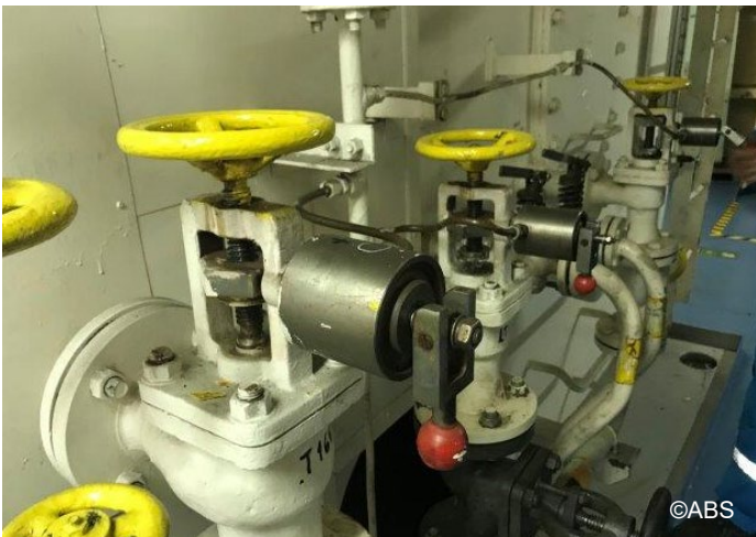
Lubrication oil system quick closing valve inoperative
