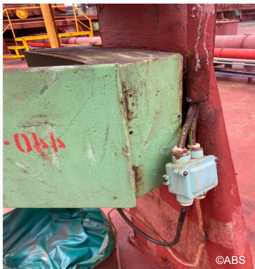
Unsecured junction boxes and cables on deck
