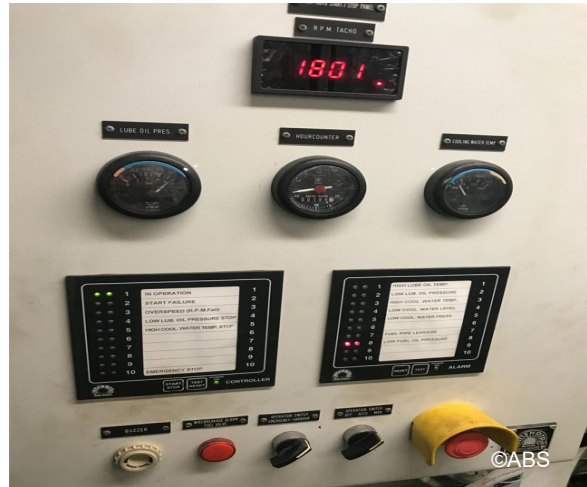
Crew not familiar with procedure to manually connect emergency generator to switchboard
