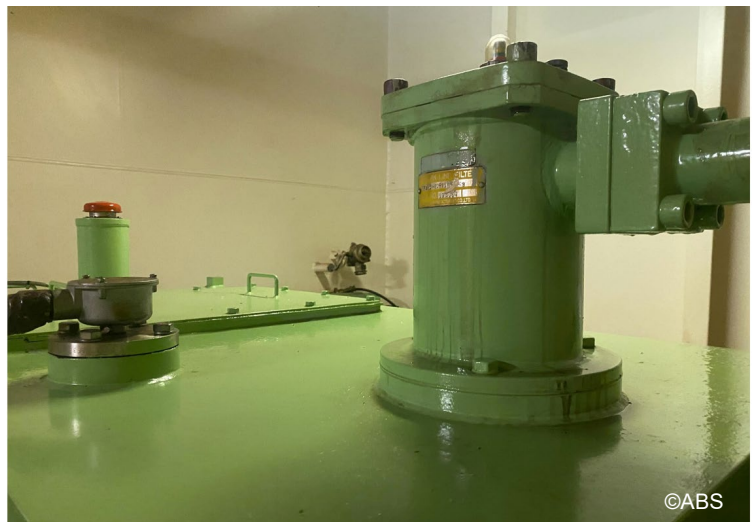
Leakage of deck machinery hydraulic pump circulating system located at Forecastle Space
