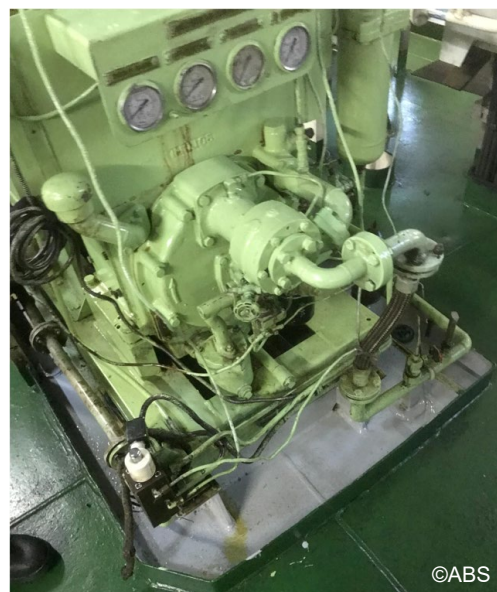
Oil leakage from main air compressor pumps
